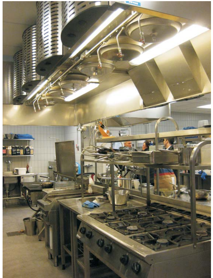
Jeven TurboSwing hoods with supply air units.
